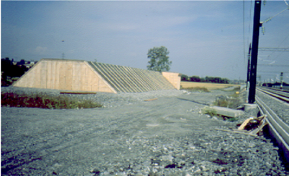
Figure 4 Test field with refrigerated building at the New Airport Express Line at Leirsund.
