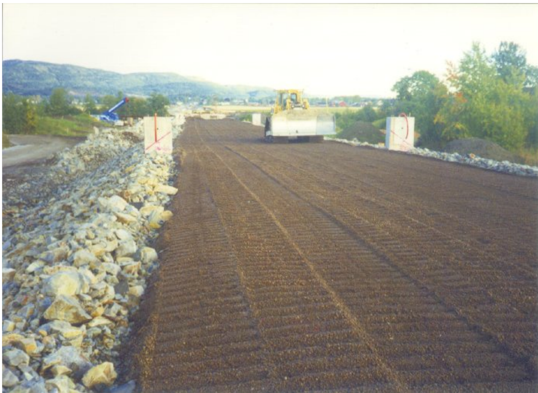
LWA used as frost insulation and light weight fill in railway embankment. Vestfoldbanen, Norway.
