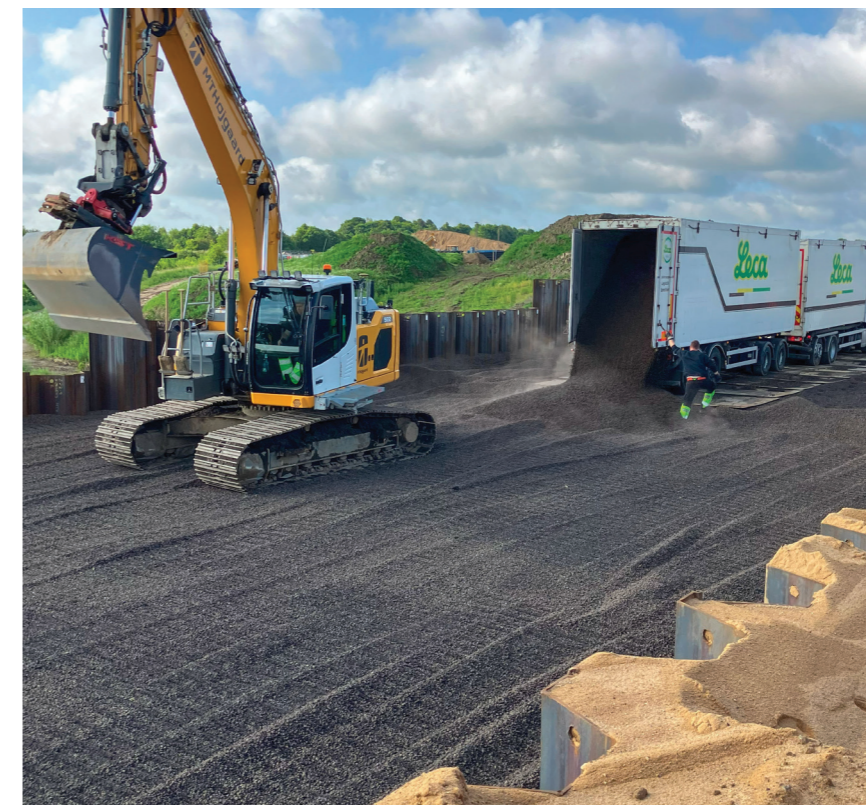
Leca® lightweight aggregate being placed on the E45 motorway — reducing load and earth pressure in the road structure.
