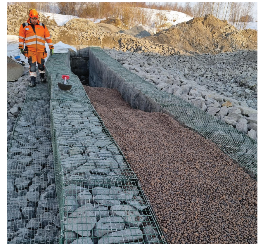
Leca LWA placed in the dam core, easy to replace.
