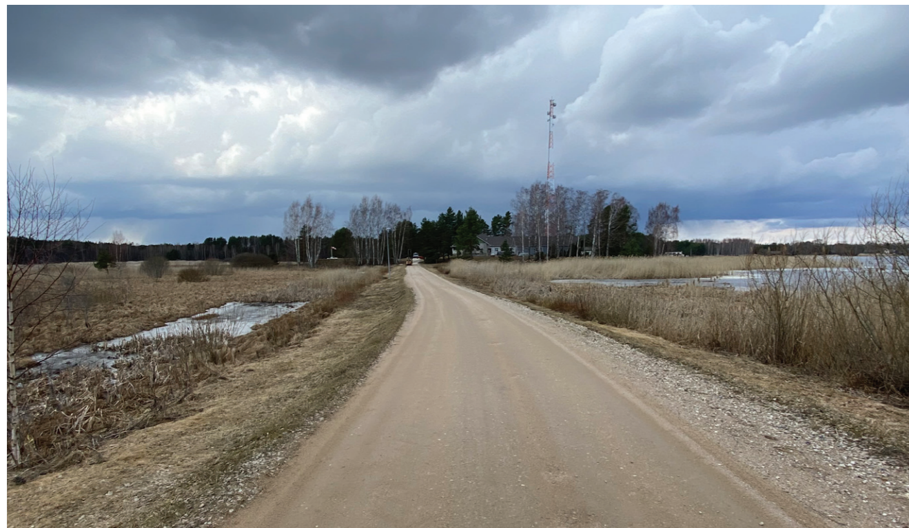
The 160-meter stretch of road leading to the Estonian Border Guard station, is still in excellent condition after over 24 years of use.
