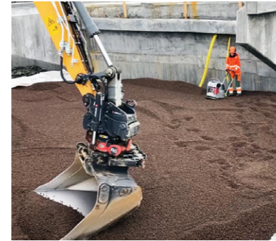
An excavator spreads Leca LWA, critical for addressing geotechnical challenges along the Lösen-Jämjö road.
