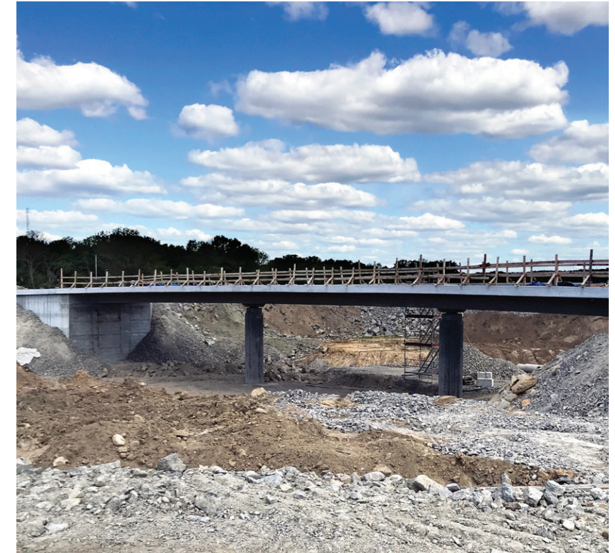
One of the 23 bridges being built to enhance infrastructure, where Leca LWA prevents additional piling.
