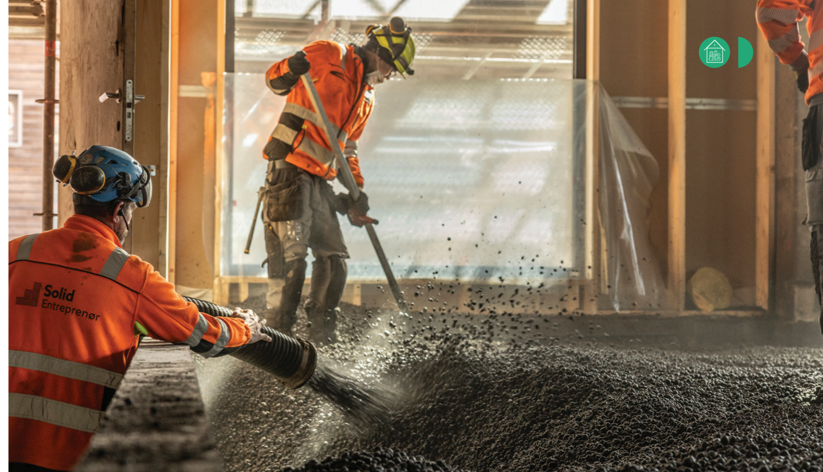
Leca LWA is blown into place directly from the truck, practically pre-compacted, with no need for manual unloading. It's hassle-free to walk on and requires zero packaging.
