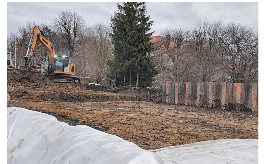
A protection of the track bed crown was constructed in the form of a retaining structure made of a sectionally anchored steel sheet pile wall.
