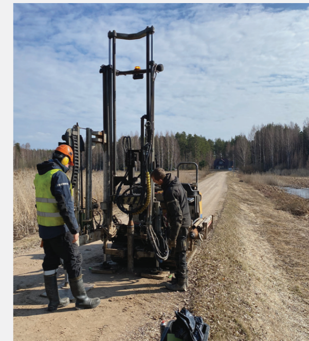
Test drilling in March 2024 to assess the condition of Leca LWA in the Varska road embankment.
