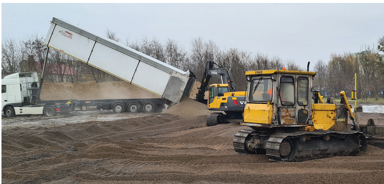
The Leca LWA was delivered by tipping truck, enabling fast and efficient installation directly on site.
