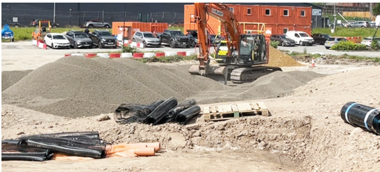
3,000 m 3 of Leca LWA used in retaining walls for a new elevated pedestrian walkway.
