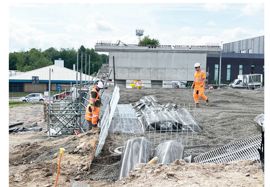
Lightweight fill required to reduce settlement risk and structural load on bridge abutments.
