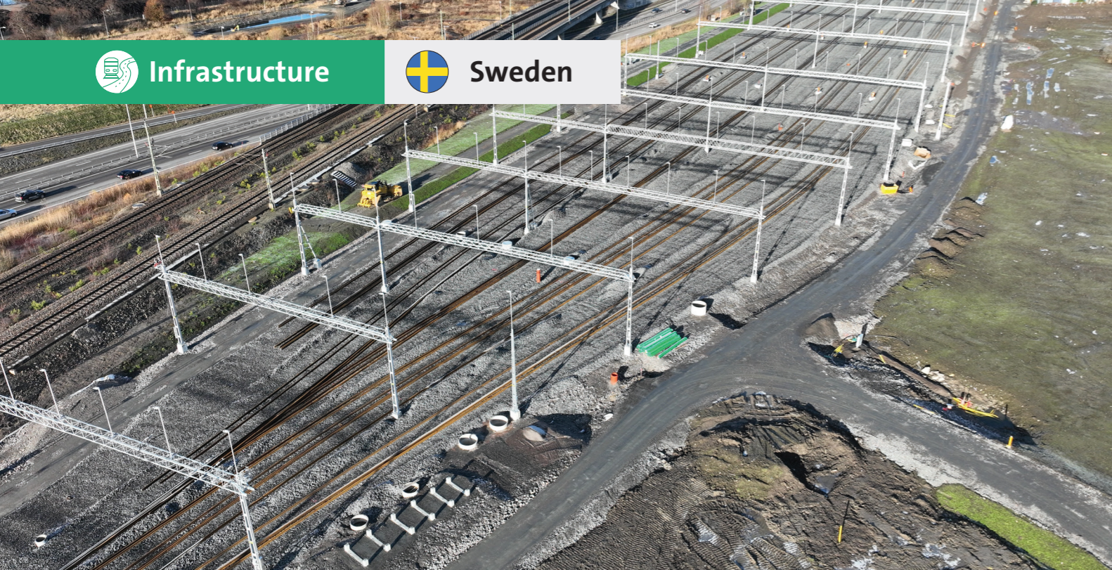
New stabling tracks taking shape – designed for increased capacity and future rail traffic. Photo Tim Cato, The Swedish Transport Administration
