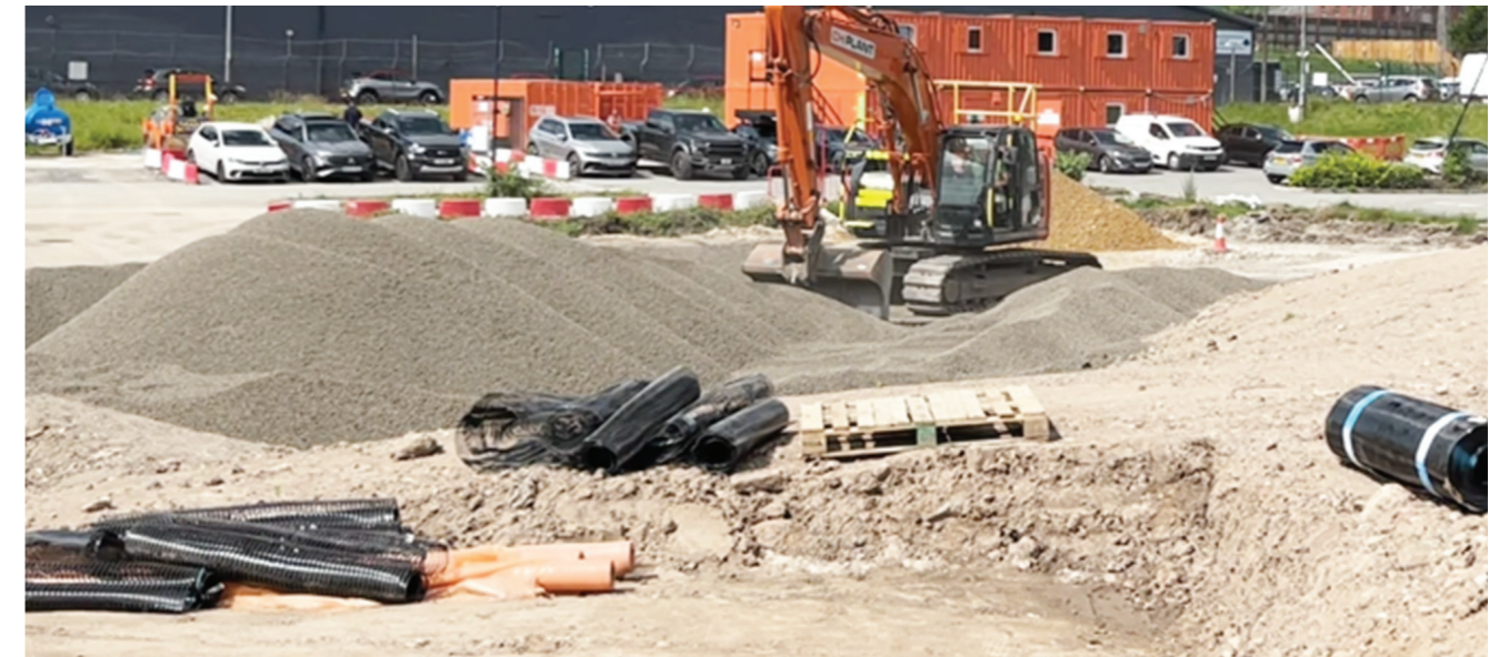
3,000 m 3 of Leca LWA used in retaining walls for a new elevated pedestrian walkway.
