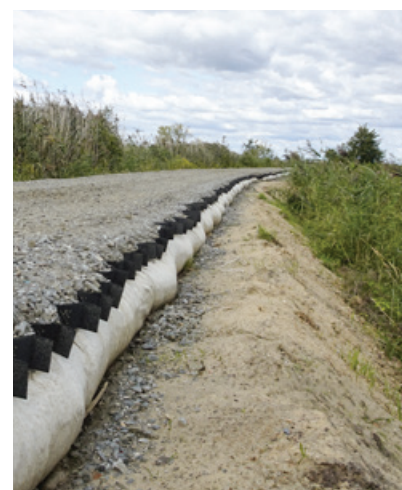
Next, a 20 cm thick surface layer made of 0–31.5 mm aggregate was laid within a geogrid.
