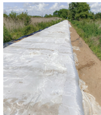
Structural fill in the form of “mattresses” made of lightweight expanded clay aggregate wrapped in geosynthetic fabric
