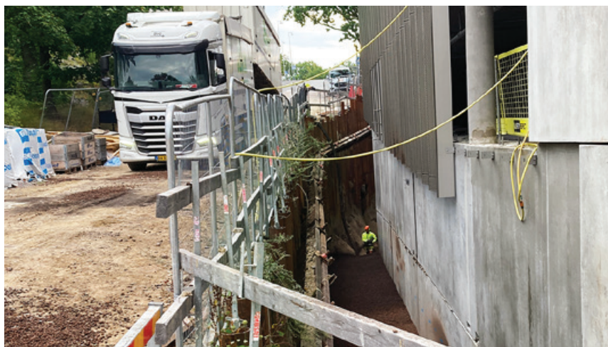
LWA is delivered by blowing to reach hard-to-access trenches at the parking structure.
