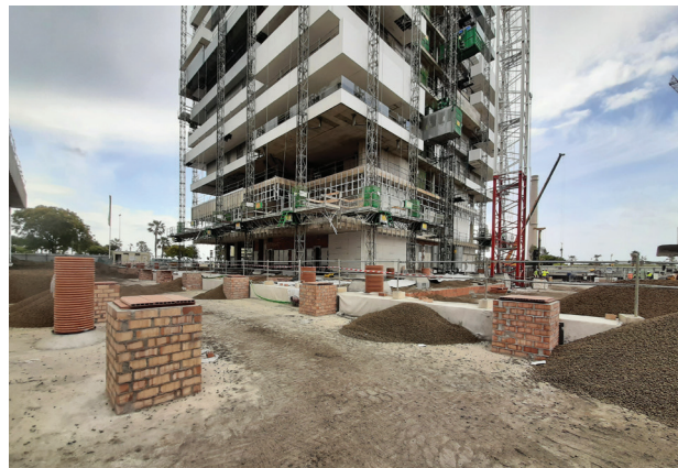
The landfill accommodates services, such as electricity, water, and wastewater
